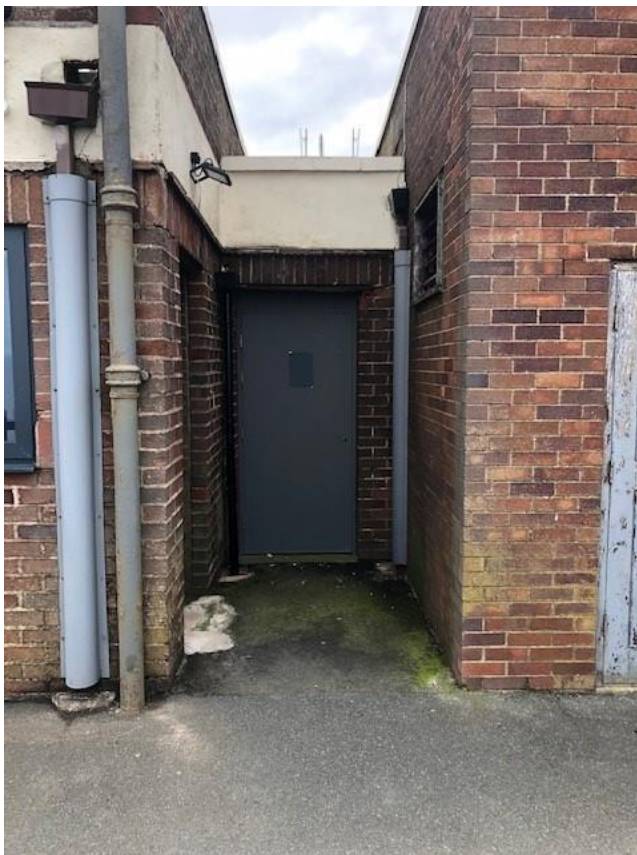
Recess between tram station building and substation building where staircase will be positioned
